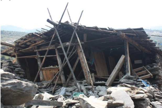
Figure 17. Collapsed house 2016 (Authors)
